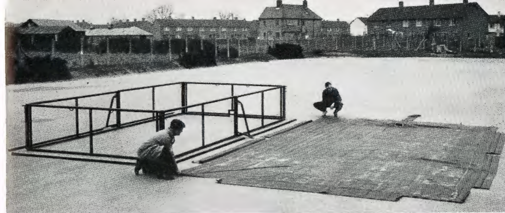
Portable pool. Southampton Education Department has developed this portable swimming pool for its primary schools. Left: The steel framework. Below: The pool completed, with the water container made from a single flat sheet of ICI 'Hydex' pvc-coated nylon fabric manufactured by ICI (Hyde) Ltd. and filled from a 6 in. 'Hydex' hose. (See also page 83.)
